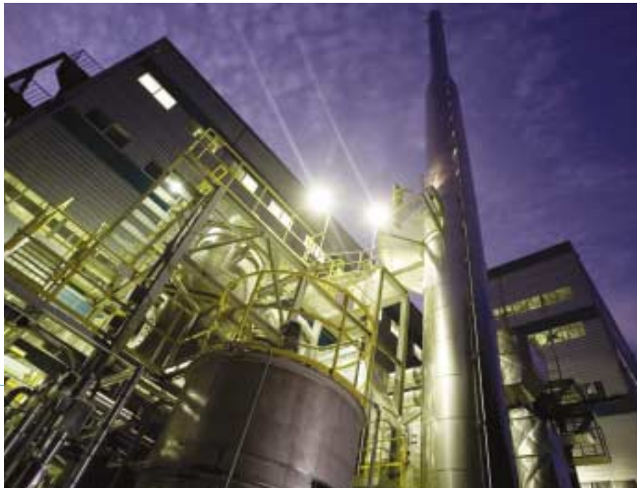
◀ 연소배가스 처리기술 종합실증시스템 (Integrated Test System for Flue Gas Treatment Technologies)
